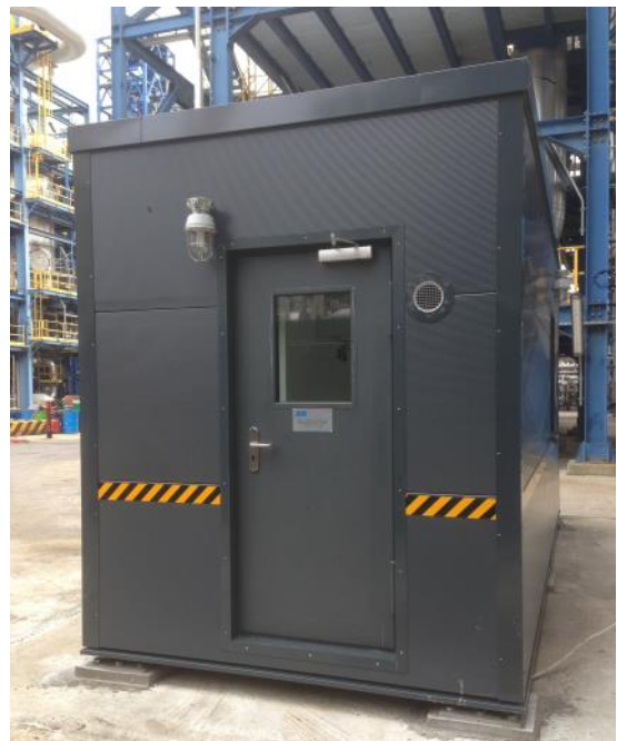
Glazed steel door with top mounted door closer.
